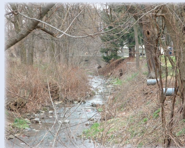
Stormwater pipes discharging directly to a stream
